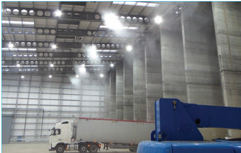
Power Station Tipping Hall - Prevents migration of Dust or Odour
