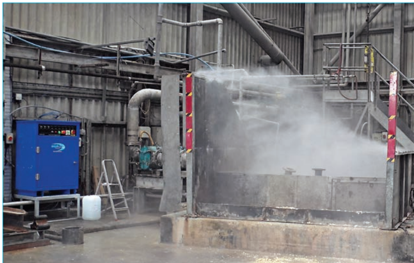
Underground storage bunker. Fog prevents dust and odour escaping when loading and unloading
