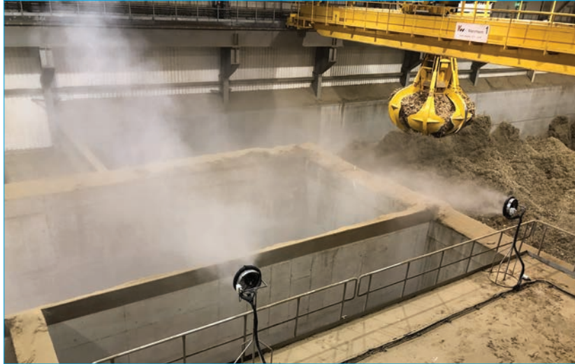
Power Station Bunker encapsulates dust and odour.
