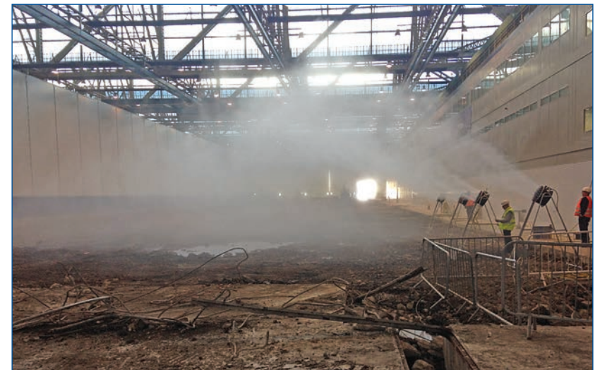
Removing and replacing concrete machine beds for Airbus, preventing dust migration to surrounding wing-manufacturing areas
