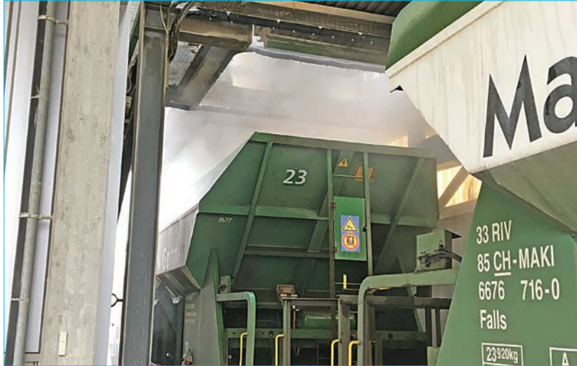
Suppressing dust when loading railway wagons
