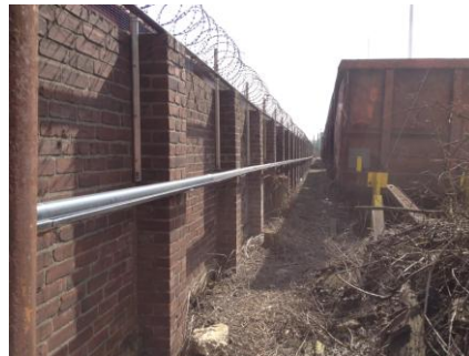
Above or below ground circulation lines around site
